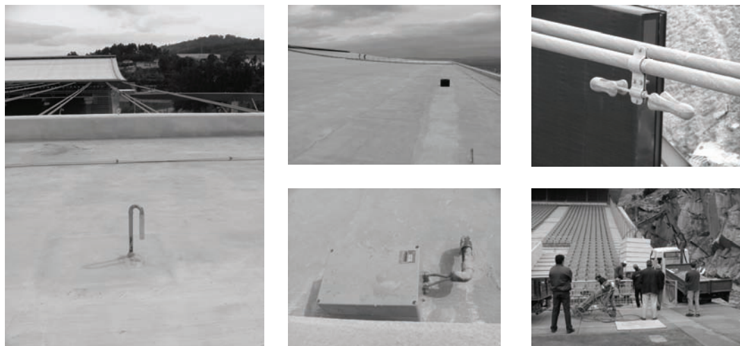
Figure 3.11 Monitoring system on the whole structure
