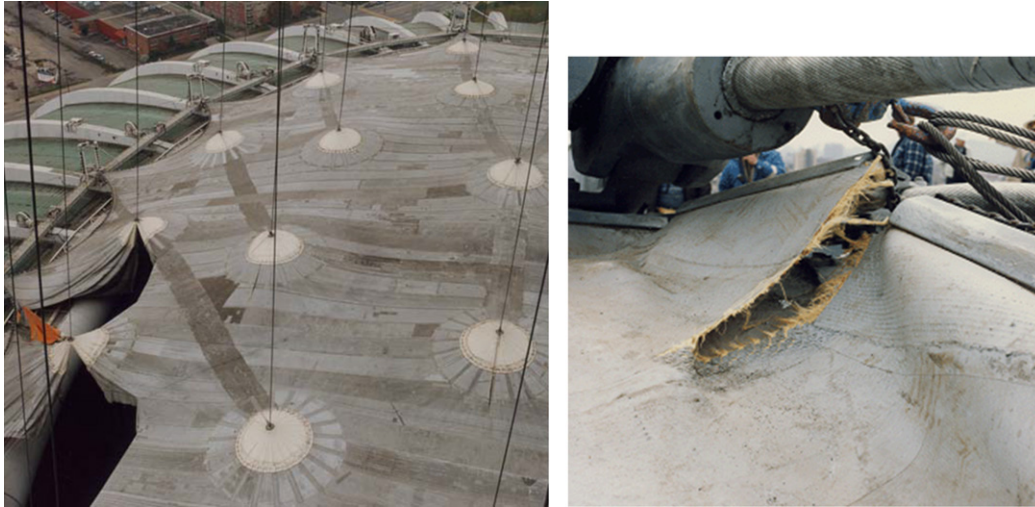
Fig. 1. Membrane failure between the suspension cones.
