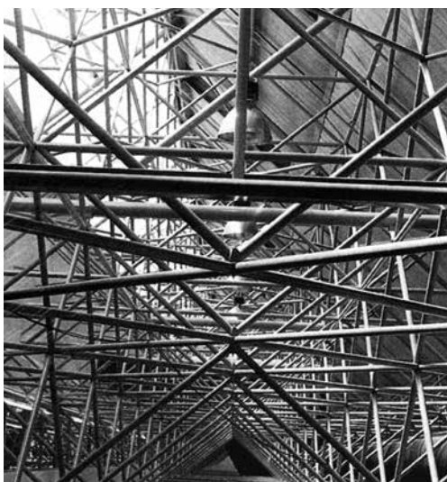
Fig. 151 Abba Space Structures, Highgate Shopping Center, reticolo multistrato Abba Cubicspace System, Johannesburg, Sud Africa, 1985
