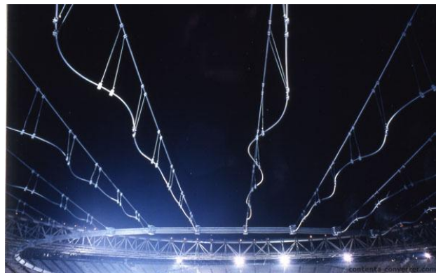
Figure 6-a: After hoisting the Tension Ring via Upper Radial Cables, prestress not yet applied
