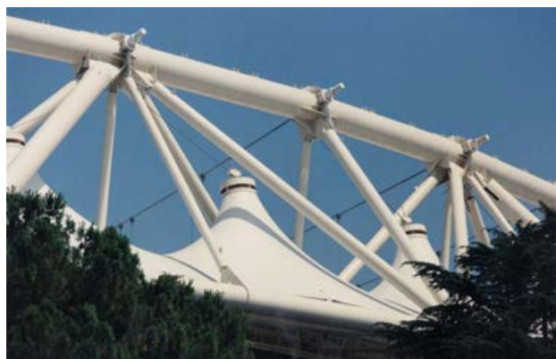
Figure 6-b: Direct tensioning of anchorage cable sockets at the backside of the Compression Ring
