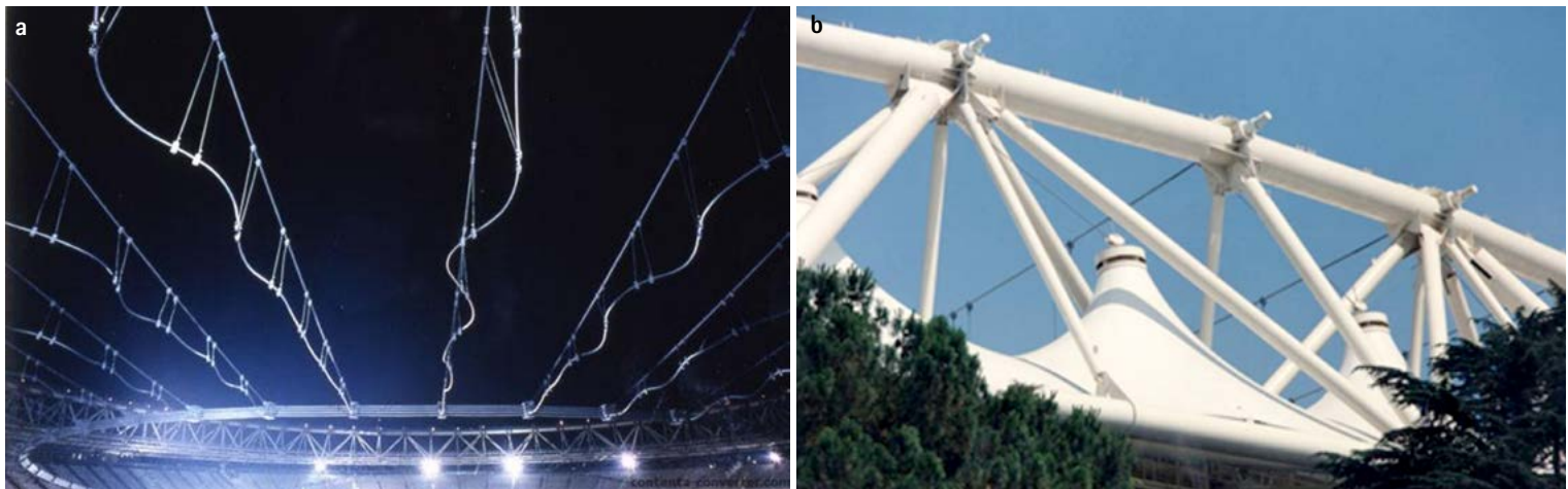
Fig. 6 - a) After hoisting the Tension Ring via Upper Radial Cables, prestress not yet applied; b) Direct tensioning of anchorage cable sockets at the backside of the Compression Ring
