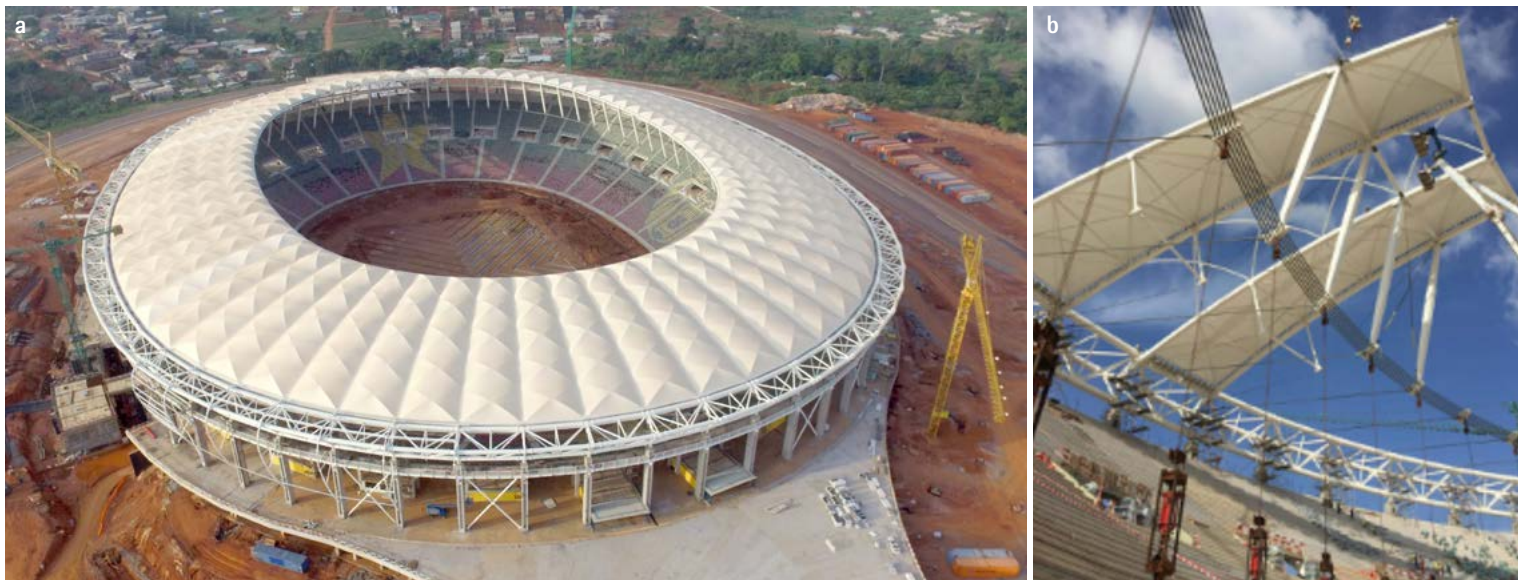
Fig. 8 - a) Aerial view of the new Yaoundé stadium; b) Installation of the hybrid radial beams
